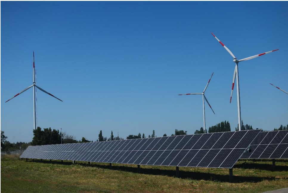
Solar parc Paillihue in Chile
